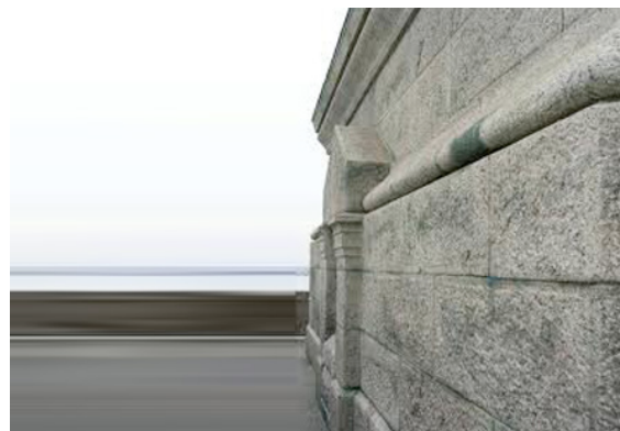
Fig 9 Copper stains on face block work
