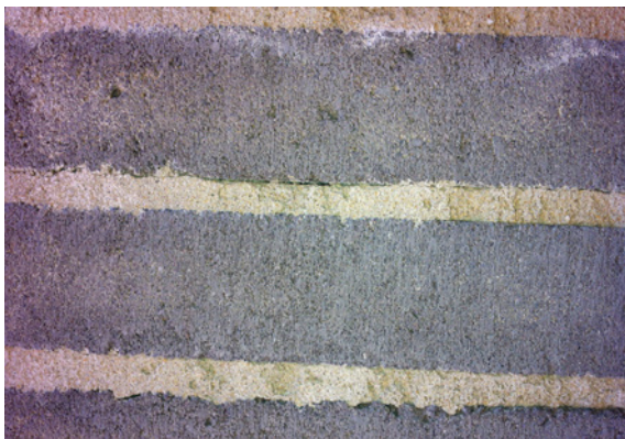
Figure 4 Damaged block wall due to incorrect use of pressure cleaning
