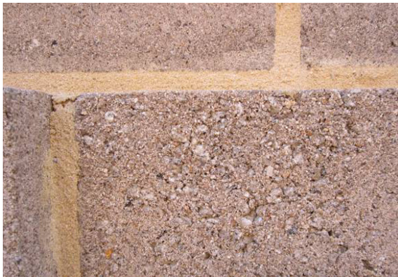
Figure 3 Damaged block wall due to high pressure cleaning
