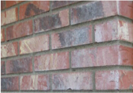
Figure 7 Calcium carbonate on face block work
