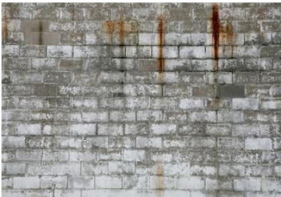
Figure 8 Acid burn on concrete masonry block
