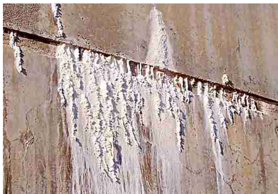
Figure 6 Efflorescence as seen on block faces (b)
