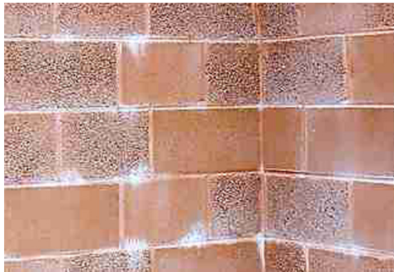
Figure 5 Efflorescence as seen on block faces (a)
